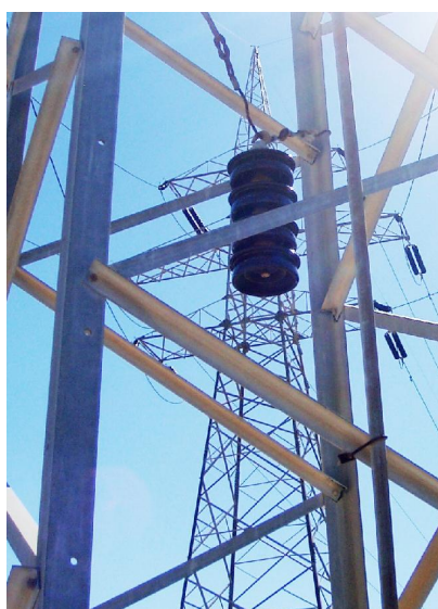
Fig. 4 A string of insulators (fog profile-porcelain) hanged (offline) from the metal structure of a 150 kV tower
